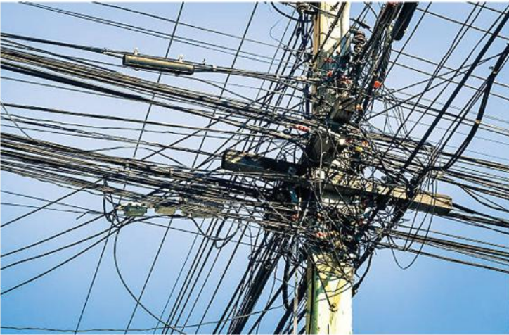
STANDARD POWER LINES IN THE PHILIPPINES
