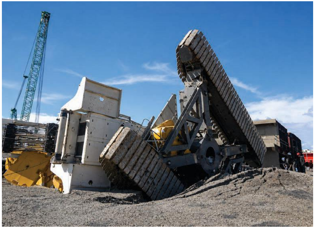
Fig. 5. Heavy rain loosens soil, causing a crane to sink into an excavation.
