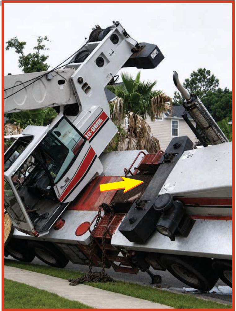
Fig. 1. Uninstalled counterweight caused the crane to tip when rotated over the side.
