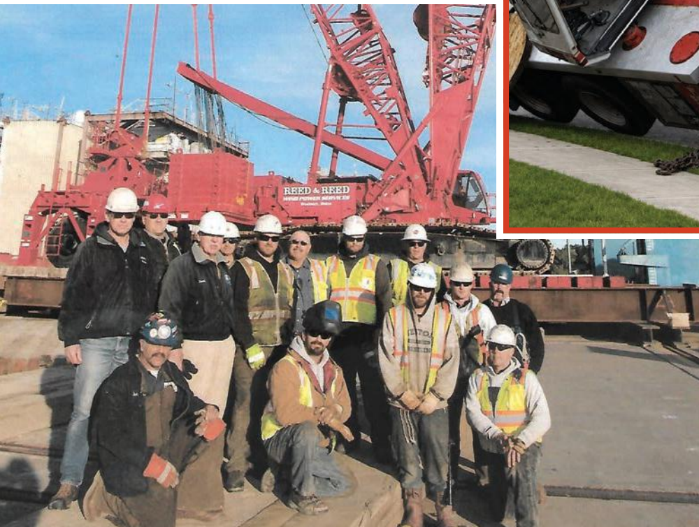
Fig. 2. This proud maintenance crew assembled this 750-ton crane on site , with the help of another 100-ton crane and crew!
