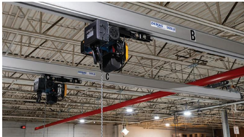
Omega Flex required a new material handling solution. Demag's KBK ceiling-mounted overhead workstation crane was selected. The installation includes 100 feet of runway across three bridges.
