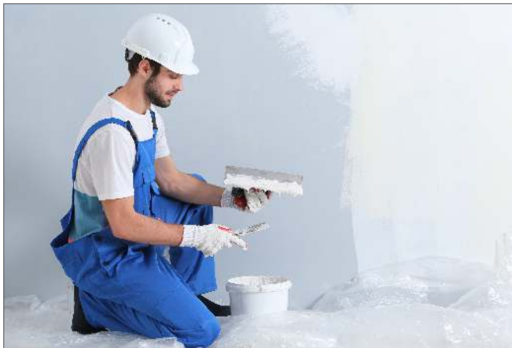
Dehumidification ensures anti-corrosion painting by maintaining temperature, relative humidity, and dew points as per technical specifications.
