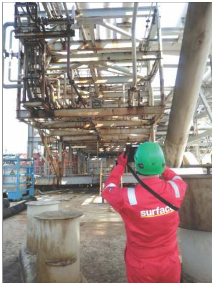
Surface Corrosion Consultants', Senior Coatings Inspector taking pictorial evidence during a conditional survey.
