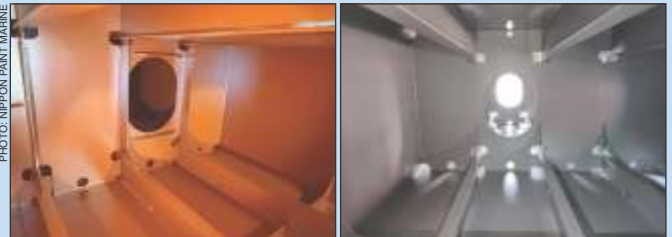
A ballast tank's first full coat of E-Marine 2000 universal primer (left) and the completed tank coating (right).
