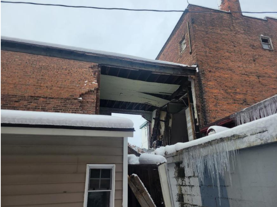
Figure 2: View of partially collapsed structure
