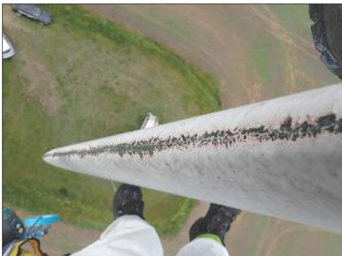
Damaged wind turbine leading edge.
