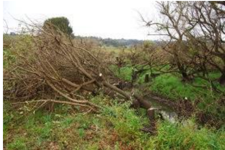
Hundreds of coral trees being removed to allow access by machinery to clear the blocked drains.
