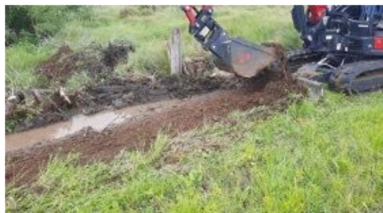
At least the digging in soft soil was relatively easy, although only suited to lighter weight machinery with the risk of getting bogged.
