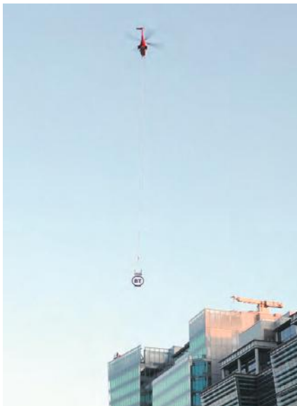
Three Snowhill, Birmingham, above and previous page: BT's Birmingham Hub at Three Snowhill in the centre of the city required UPS, batteries and chillers lifted to the roof to
