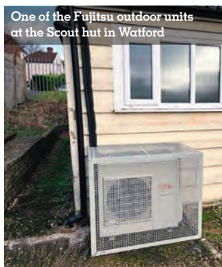
Two indoor units provide heating for the group, with the added bonus of cooling in summer
