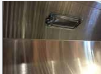
Interior Halogen Lighting
