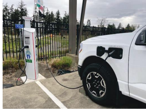
1 of 9 EV charging stations installed across 3 PPW facilities in 2025.
