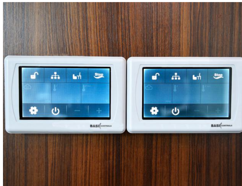
The meeting rooms and offices are equipped with occupancy sensors which activates the air-conditioning when motion is detected.
