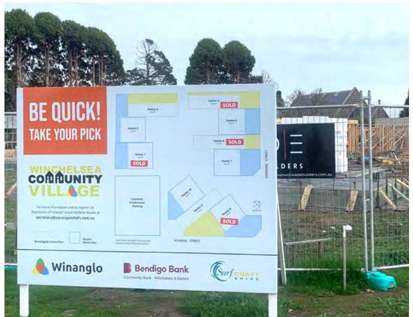
The building phase is well under way thanks to Wade Builders and their team.
