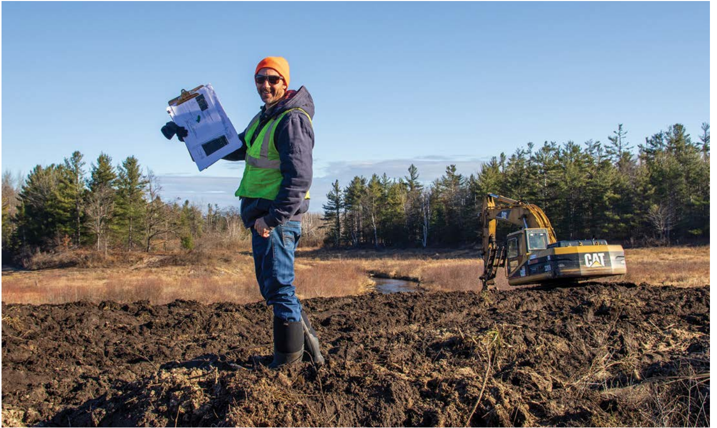
CRA Project Manager Tom Vitale oversees wetland restoration work as crews shape the landscape behind him.
