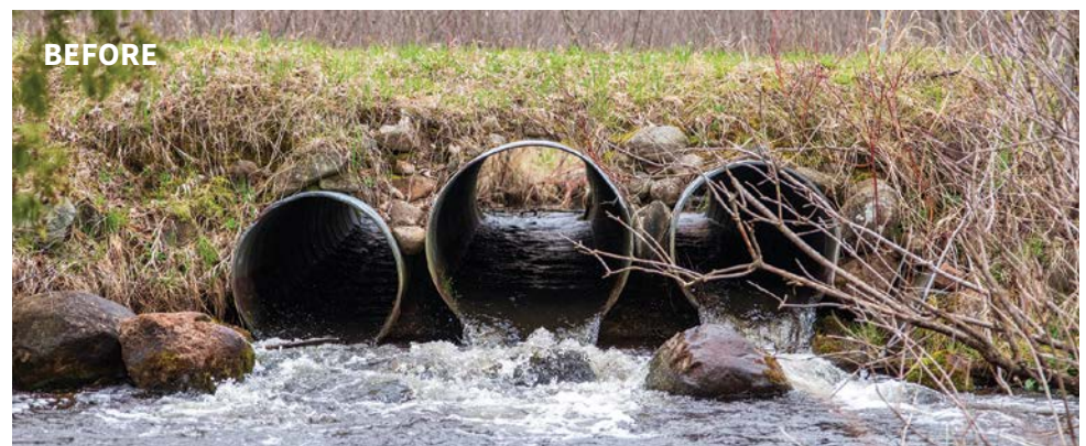
BEFORE The former culverts were elevated above the channel, restricting fish passage and causing sediment to accumulate upstream.
