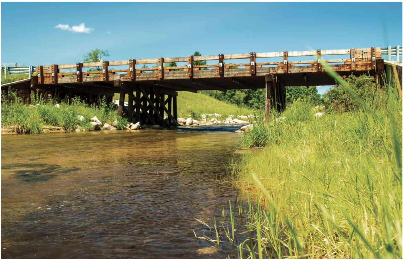
The timber bridge at Woodland Road, just downstream of the former Lake Kathleen Dam site, was one of several projects completed as part of the Initiative.
