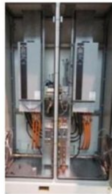
Compressor drives + main power connection
