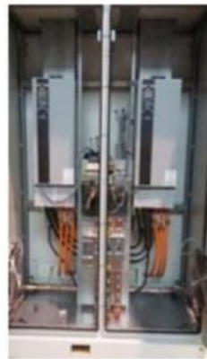
Frequency converters compressor drives + main power connection
