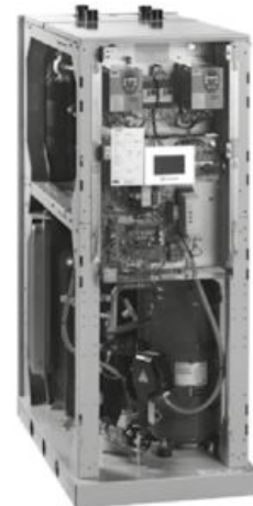
Access to control panel
