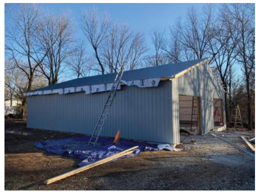
This is how it stands at the time this went to press. Four walls and half a roof. I will take you through the trials and tribulations of the build in the next installment.
