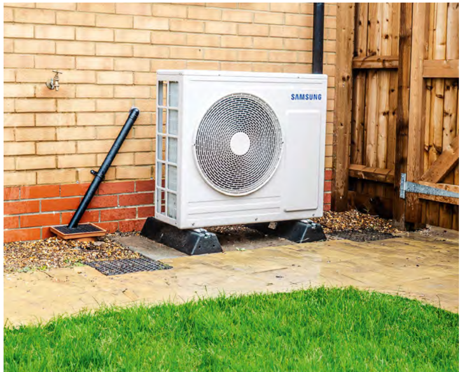
An installed Heat pump in Glenvale Park
