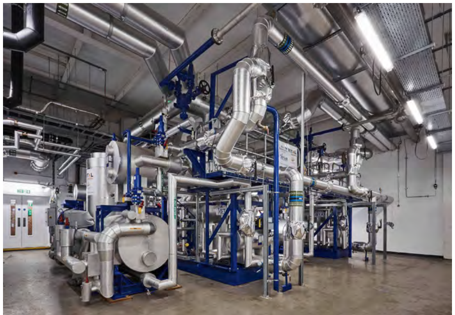
Vital Energi - Queens Quay Water Source Heat Pumps
