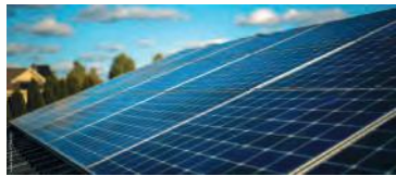
17 solar PV panels
