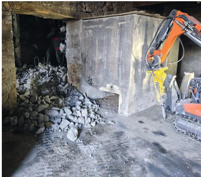
Colum and Aidan plan to renovate the house and have already begun demolition
