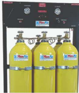
Air Storage Cylinders
