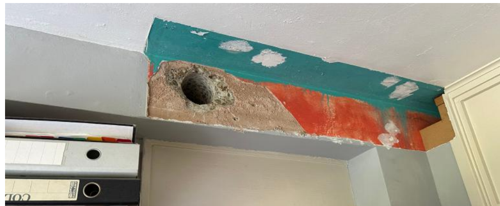
Example of a home where the MVHR ventilation system has been stripped out, with ductwork routes still visible but no replacement ventilation system has been installed.
