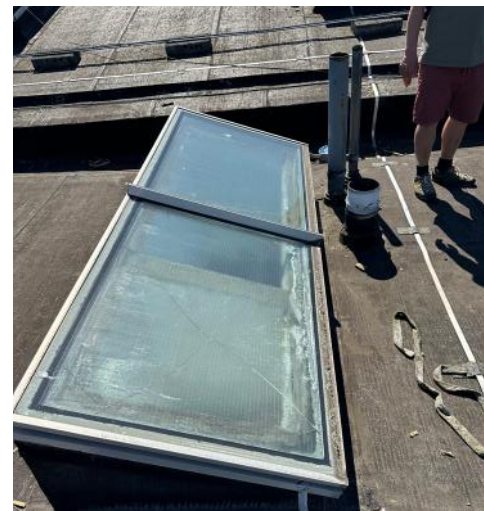
Multiple potential air leakages through the roof of Bence House including service penetrations and defective single glazing in the rooflights.
