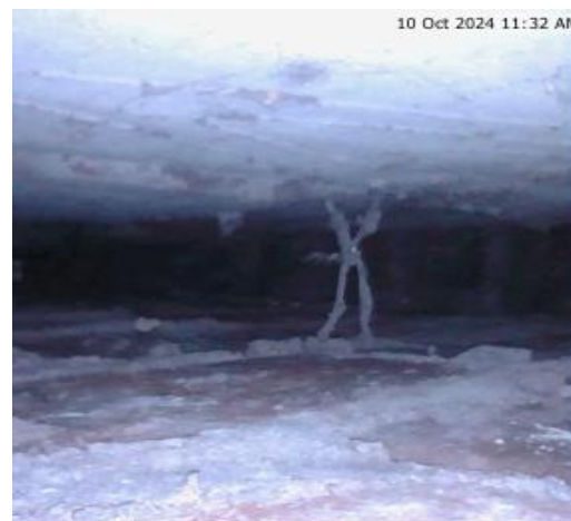
An example of a borescope image taken as part of a retrofit assessment of a property with cavity wall construction, in this case showing the wall ties and that there is no insulation present within the wall cavity.
