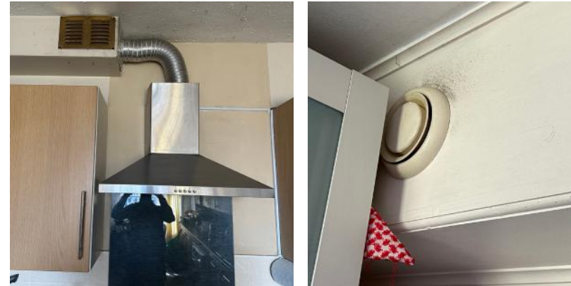
(above left) A kitchen extractor connected to an MVHR system and (above right) a supply air register in the same property with black discharge.
