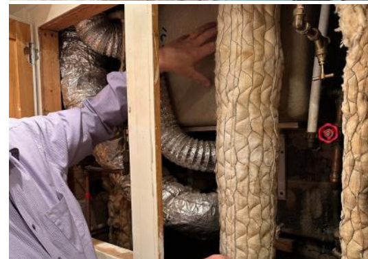
A service duct within a Type B scissor flat WC containing numerous active services (including water and waste pipes) and defunct services (including district hot water and ventilation).
