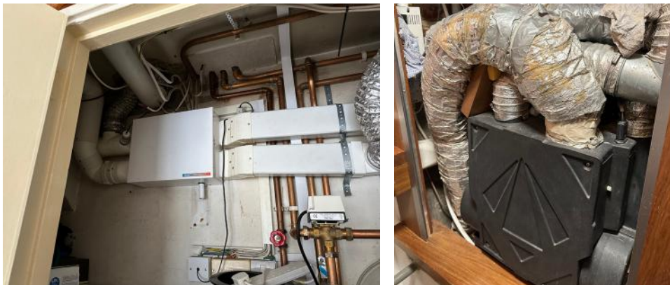
Examples of MVHR installations in Bence House: (left) In the kitchen service riser within a Type A maisonette; (right) In the WC service riser within a Type B scissor flat.
