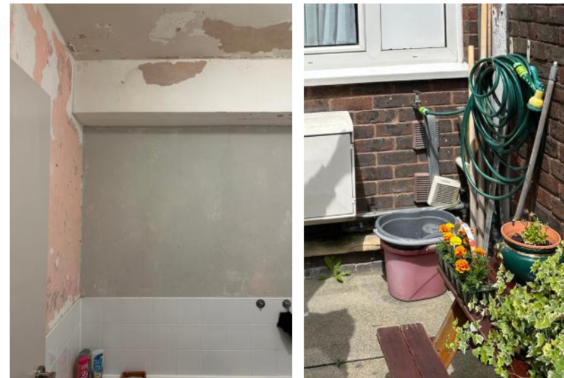
(above left) Evidence of condensation and moisture damage within the bathroom of a property with a non-functioning MVHR installation; (above right) Intake and exhaust MVHR vents situated too close together in an external wall.
