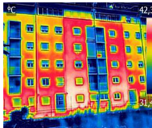
An example of a thermographic imagery of a building showing heat distribution across a façade. Note the impact of thermal bridges around window openings and balconies.
