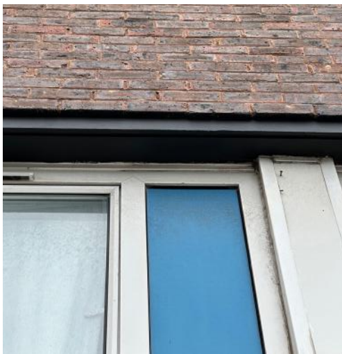
Part of the concrete structure at Bence House penetrating the building envelope over a window forming a localised 'cold' thermal bridge between the interior and exterior
