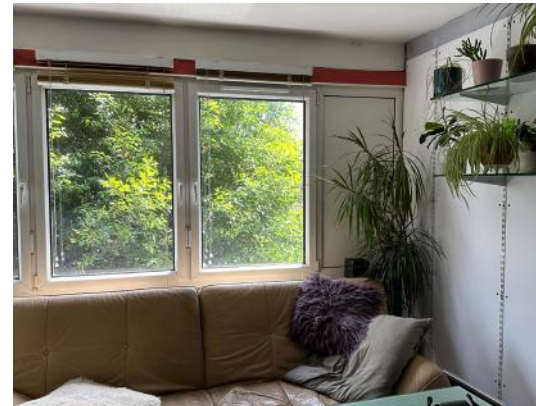
Typical windows and solid spandrel panel, in this case within the living room of a Type B scissor flat. The windows are non-original, PVCu, double glazed units with trickle vents.
