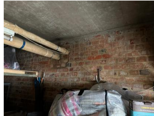
A garage interior with the solid floor slab of a Type A unit above (upper level bedrooms). There is an opportunity to consider insulating this floor slab from below.
