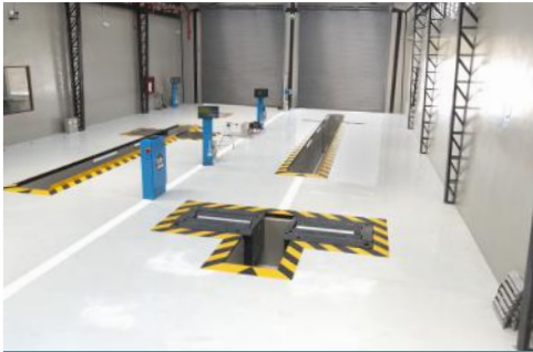
LV | HGV FULL TEST LANE
