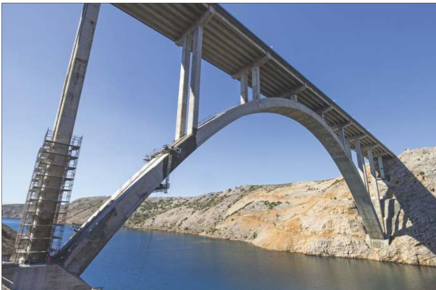
The only answer is to build structures in a way that will slow down the corrosion process and thereby extend service life.
