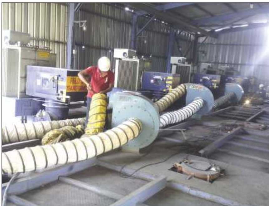
Humidity and temperature control system on rent for quick drying requirement.
