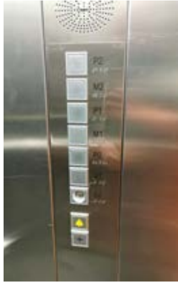
Ascensor C / Elevator C
