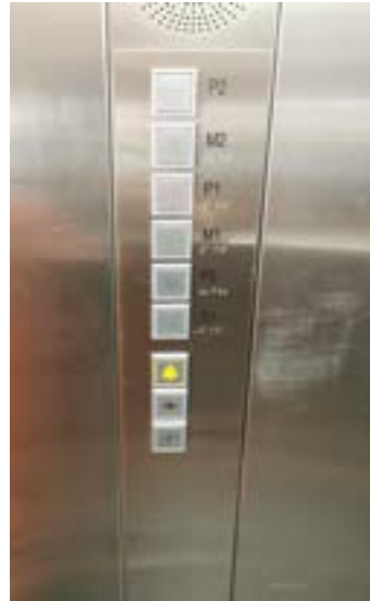
Ascensor B / Elevator B
