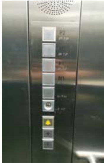
Ascensor D / Elevator D
