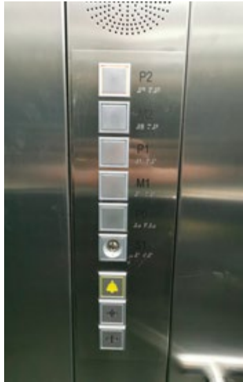
Ascensor D / Elevator D
