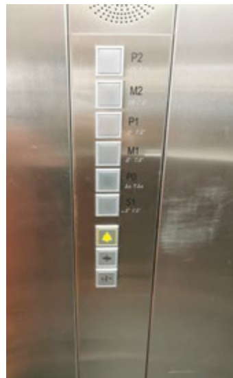
Ascensor B / Elevator B
