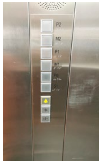
Ascensor B / Elevator B
