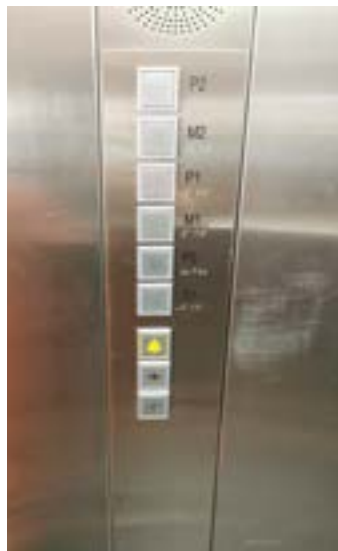
Ascensor B / Elevator B
