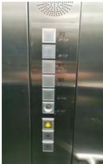
Ascensor D / Elevator D
