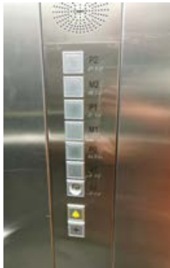
Ascensor C / Elevator C
