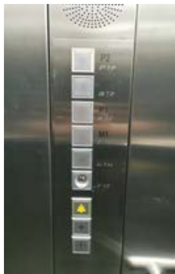
Ascensor D / Elevator D
