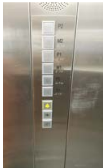
Ascensor B / Elevator B
