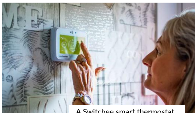
A Switchchee smart thermostat
