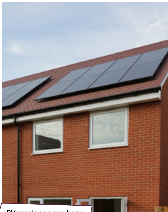
PV panels on a new home
