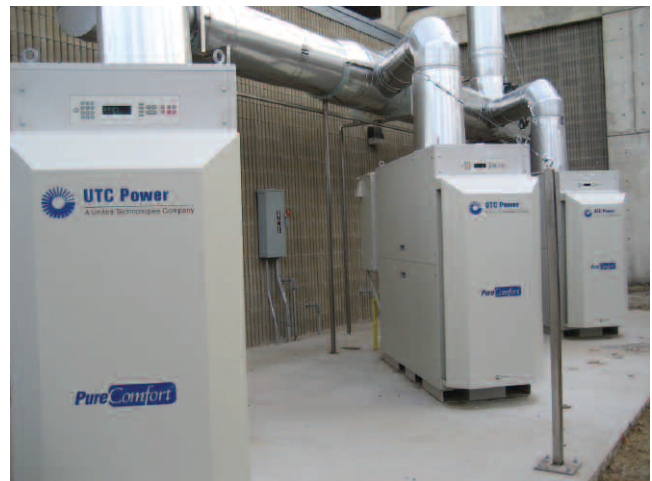
High-efficiency microturbines provide heating, cooling and electricity for the TAC building. An interactive display of the system's efficiency is located in the lobby.
