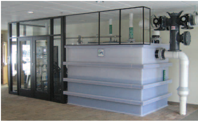
The rain-harvesting system is located in the building's naturally ventilated lobby.
