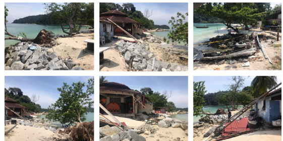
Figure 3 Erosion and the damages to the coastal infrastructures at Coral Beach
