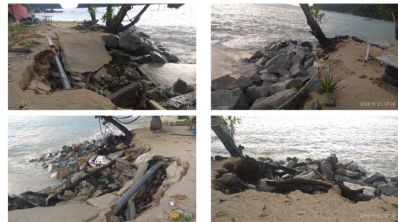
Figure 2 Failure of the existing rock revetment
