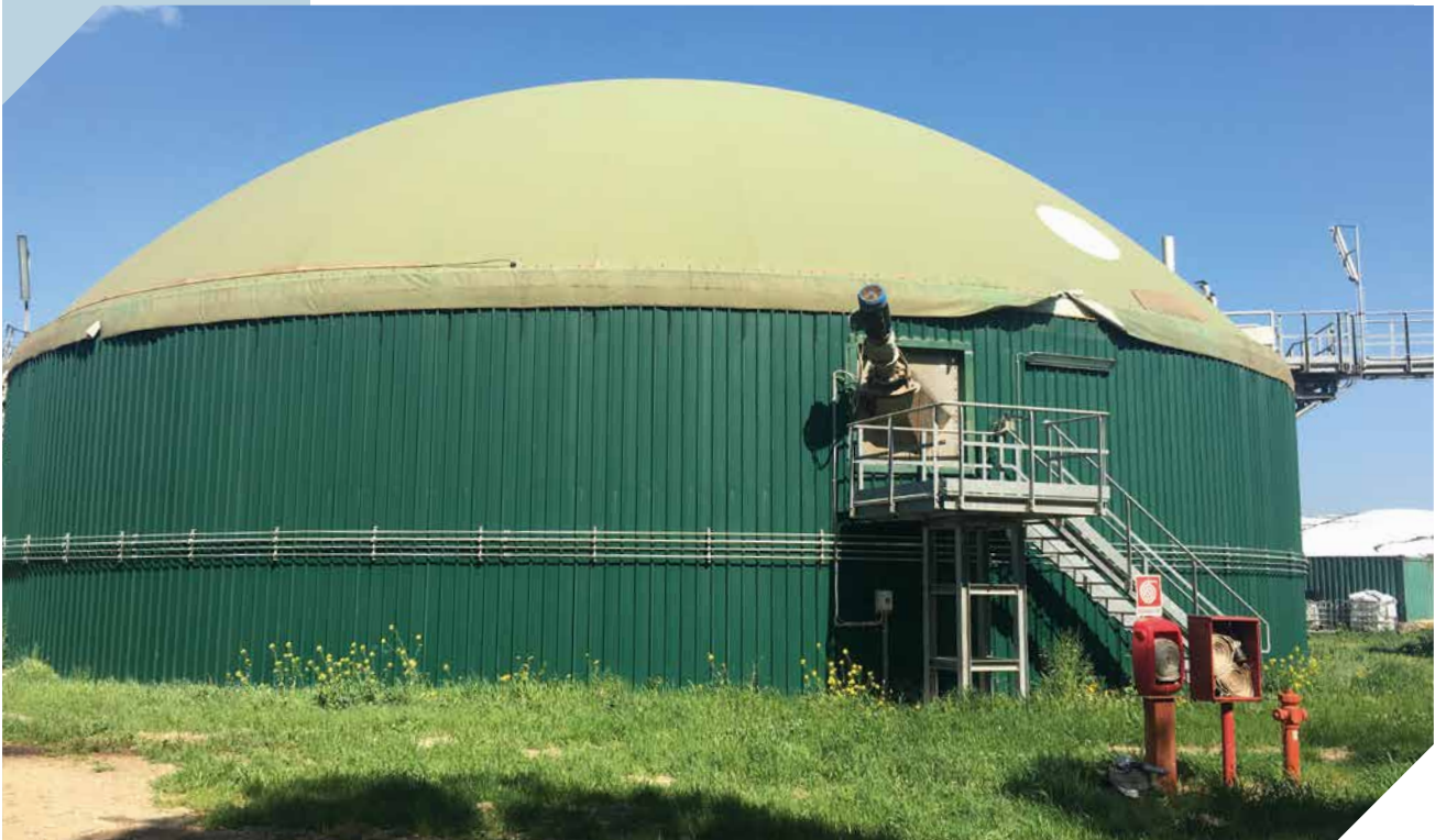
Decimoputzu Biogas Plant
