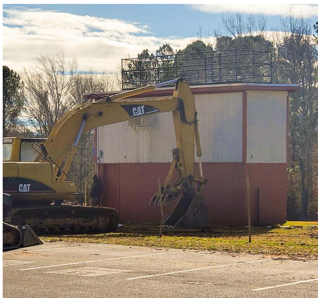
The press box at Abbeville High School was recently demolished, and there are plans to build a new one. (Staff courtesy of Benji Greeson)
