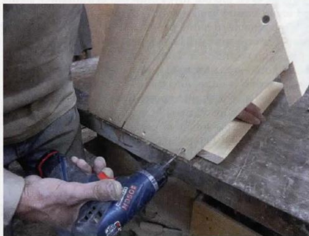
Attach the other end. See how the sides stick down below? Use your entrance reducer or a 1/8" stick to get the proper spacing.
