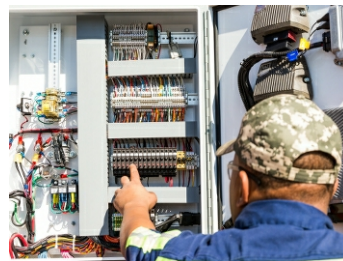
Easy Access to Heavy Duty Circuit Breaker Panel and Breaker Reset Switches
