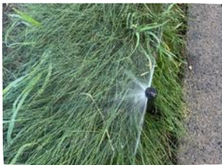
Fixed Spray Nozzles
