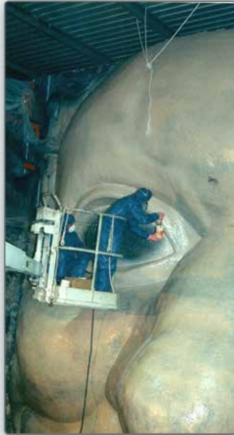
Stage 2 - Sculpting the Eye showing men working from Boom lift. - Note the enormous size of this entry statement.
