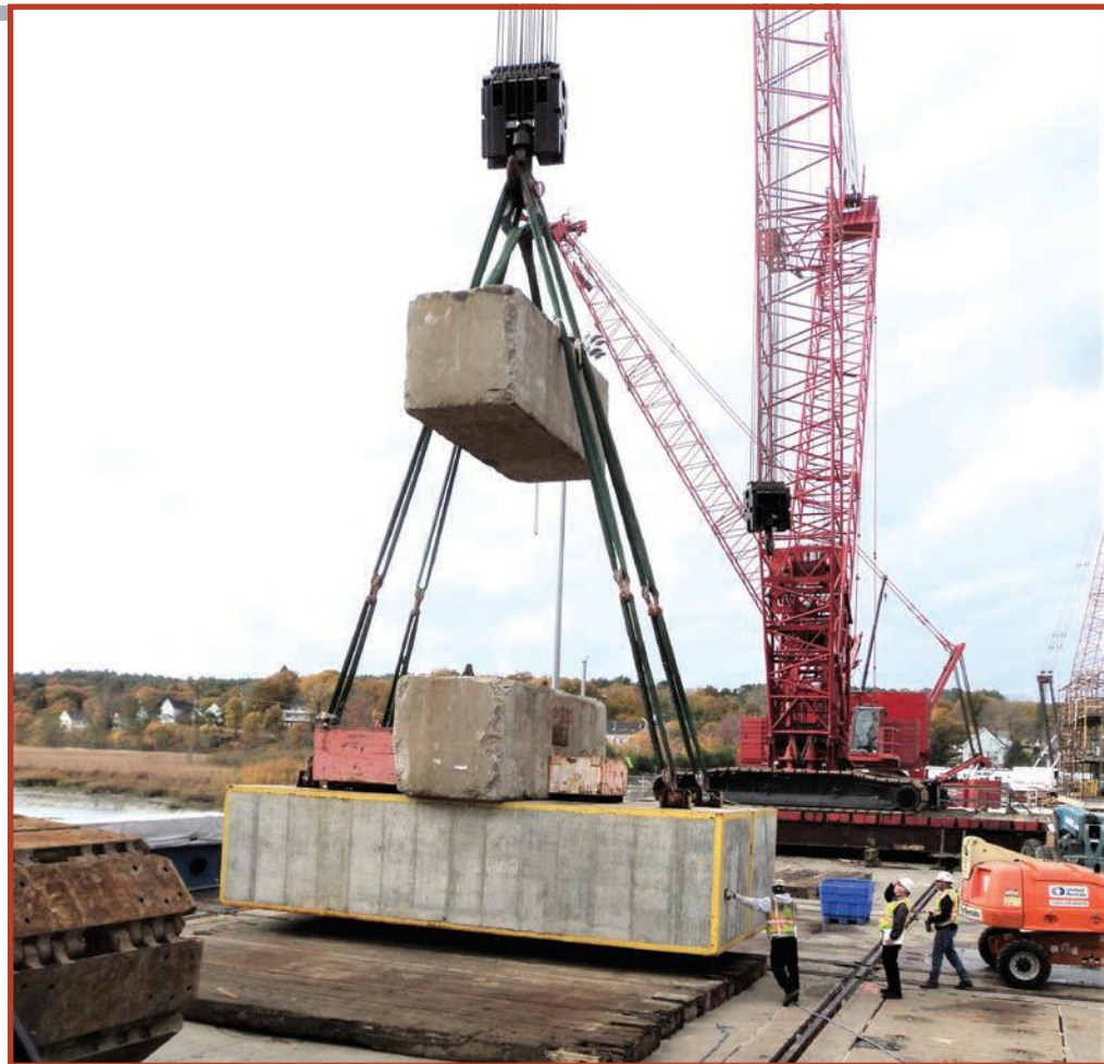
Fig. 1. All the impact forces of a moving load must first be absorbed by the hook!
