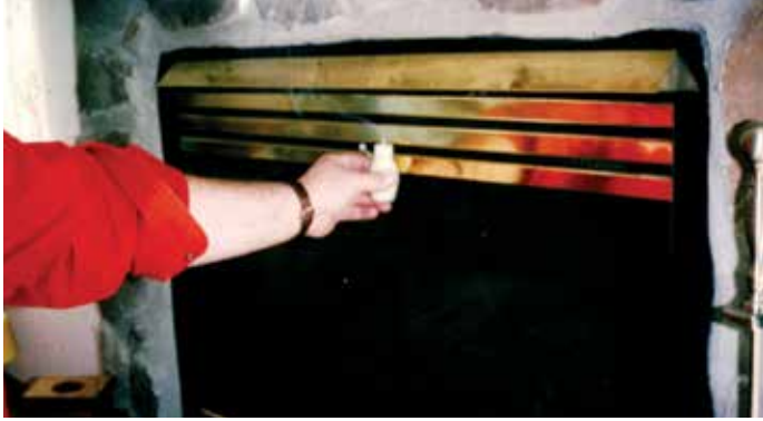
Photo 5: Back-drafting fireplace – Negative pressures due to air exhausting systems backdraft combustion systems such as fireplaces.
