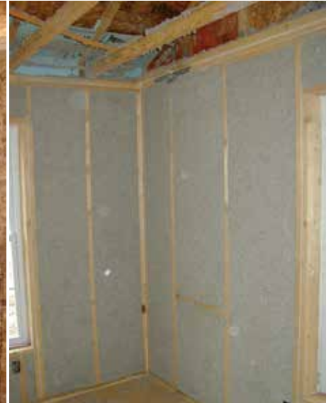
Photo 2: Thermal insulation – Significant increases in thermal insulation added to wall assemblies, roof assemblies, and foundation assemblies.
