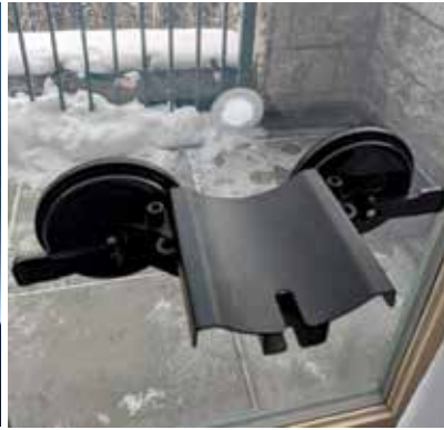
Examples of failed IGU (note: condensation between glass panes).
