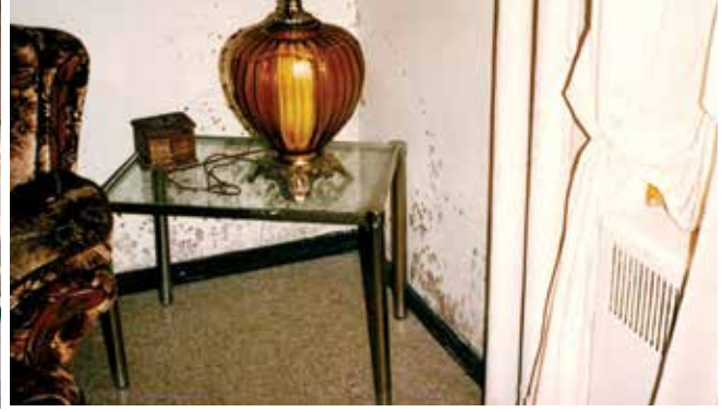
Photo 6: Mould – When we caulked and sealed old buildings, we reduced air change and increased interior mould.
