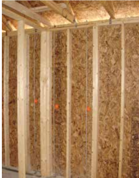
Photo 1: Moisture sensitive materials – The newer materials are by and large more sensitive to water damage than the older traditional materials. Oriented Strand Board (OSB) is significantly more moisture sensitive than plywood.
