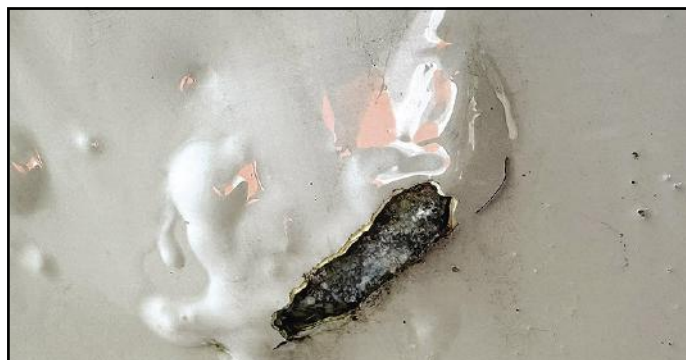
Corrosion as seen on OJA.
