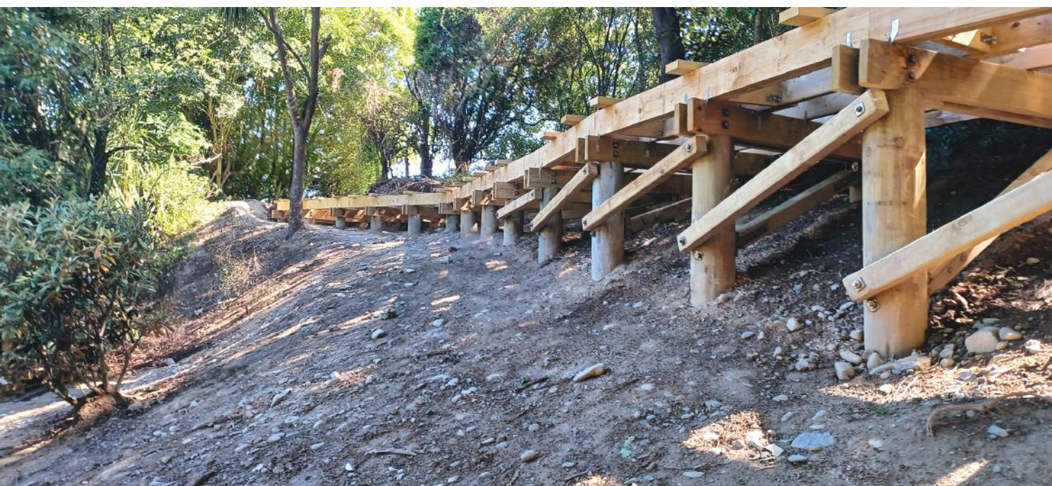
CONSTRUCTION OF THE GERALDINE SCULPTURE TRAIL BOARDWALK , alongside the Waihi River, is well underway. While pictures of the new pathway have received a mixed reception on social media, for the most part it seems the community are appreciative that the trail is now more accessible. PHOTOS: Craig Matheson
