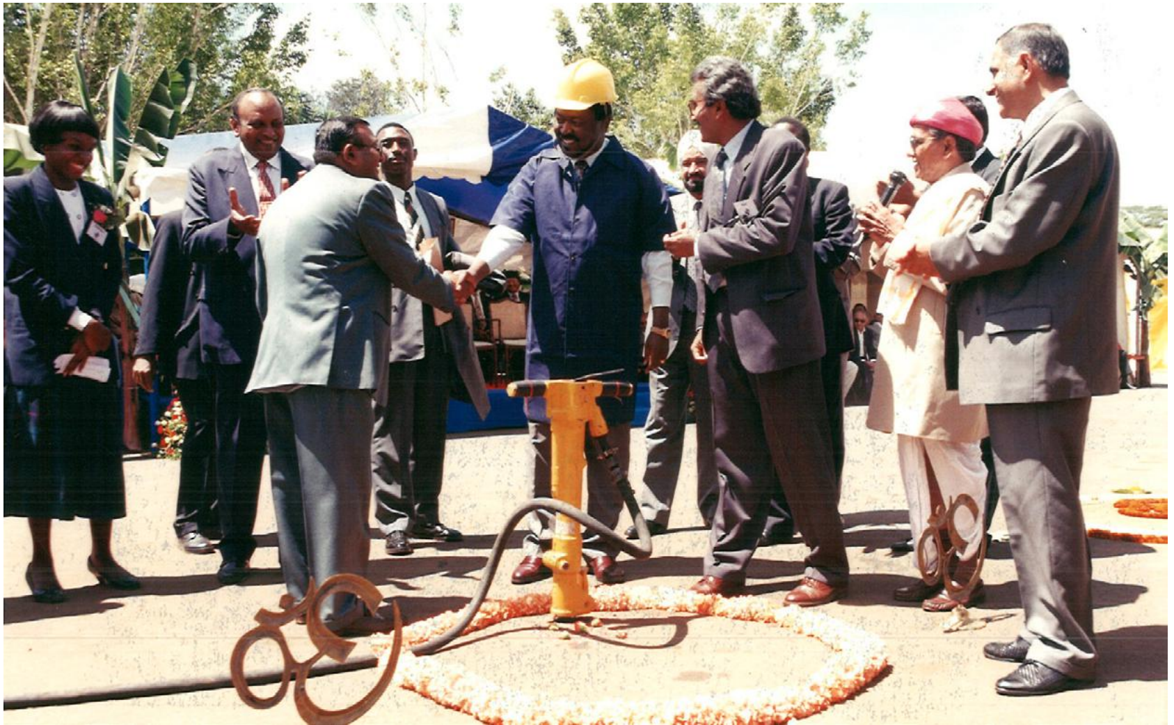
Hon. Musalia Mudavadi being requested to break ground for Phase 2, Sarit Centre.
