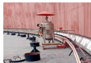
Automatic Heat Detection Cum Fire Extinguishing System For Rim Seal Area Of Floating Roof Storage Tanks
