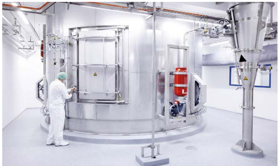
View of the centre section of the spray tower
