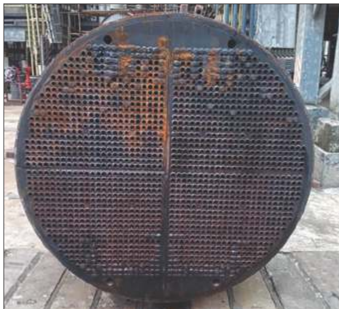
Example of corrosion of tube sheet in heat exchanger.
