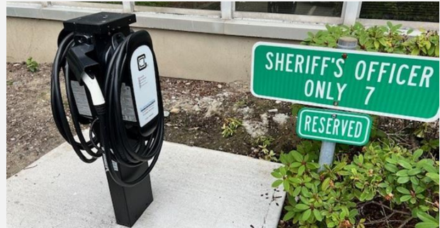
Facilities Management completed the installation of a dual head EV charger at the Sheriff's Department Headquarters at the CCB in preparation for the arrival of the Mach-E EV's.
