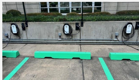
Facilities Management replaced outdated EV chargers behind the County-City Building in preparation for additional Fleet EVs.
