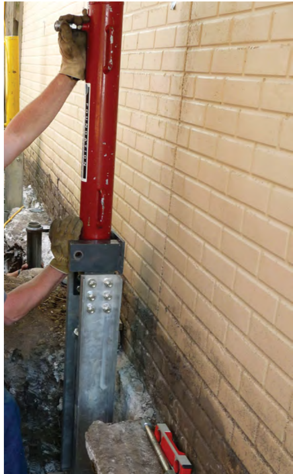
Figure 2.28 Hydraulic drive cylinder placed within top fixture of drive stand
