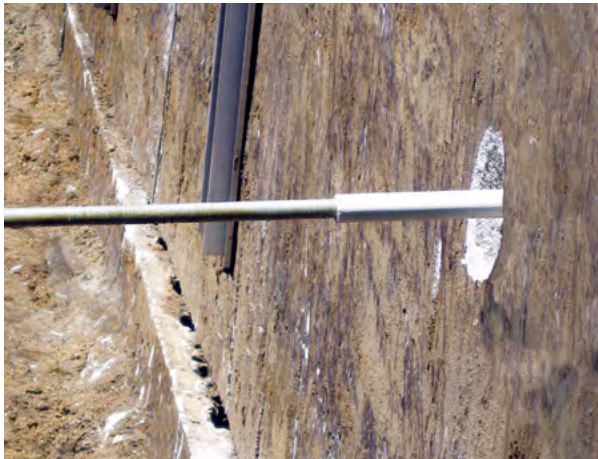
Figure 3.11 Before: Shear movement of a block wall evident from exterior
