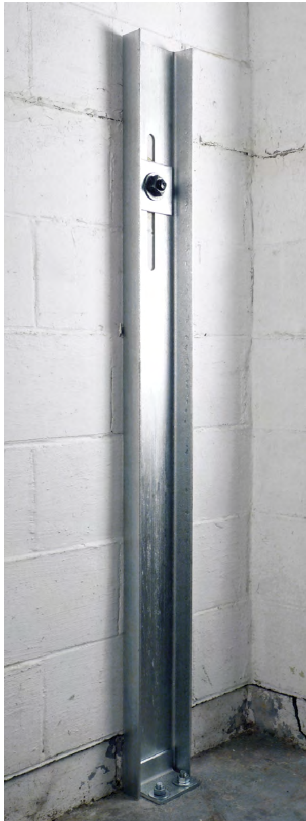
Figure 3.13 GeoLock channel anchor system installed to prevent shear movement
