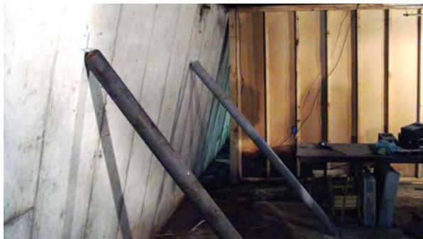
Figure 3.9 Before: Poured concrete basement wall severely leaning in at the top
