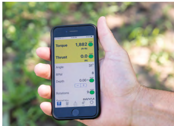
Figure 1.87 (Top) Torque transducer providing direct reading of torque for helical pile project at Reagan National Airport (Bottom) Real-time installation data being logged on an iPhone
