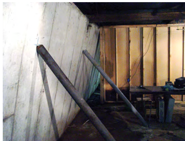
Figure 3.2 Poured concrete walls often lean in at the top and show less cracking in the interior portions of the wall
