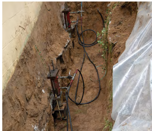
Figure 2.40 Hydraulic system connected to provide uniform application of load
