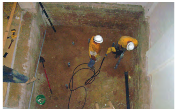
Figure 1.34 Helical piles installed with hand-held equipment to support new elevator within existing school
