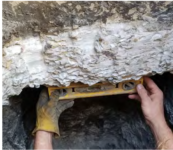
Figure 2.47 Prepare bottom of footing with chipping hammer, as necessary, to create a flat and level surface
