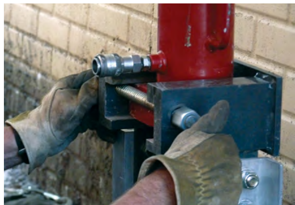
Figure 2.29 Drive cylinder locked in position with coil rod and nuts
