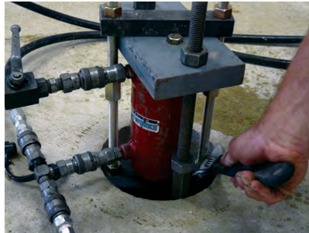
Figure 2.80 Pier load locked off by tightening nuts on top of pier cap
