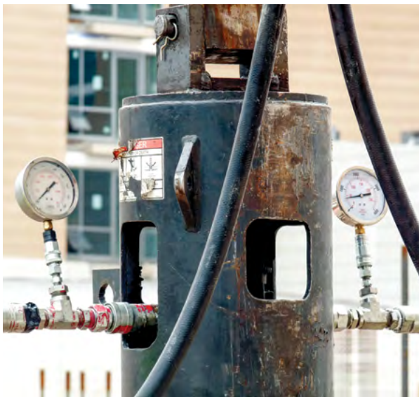
Figure 1.81 Dual pressure gauges
