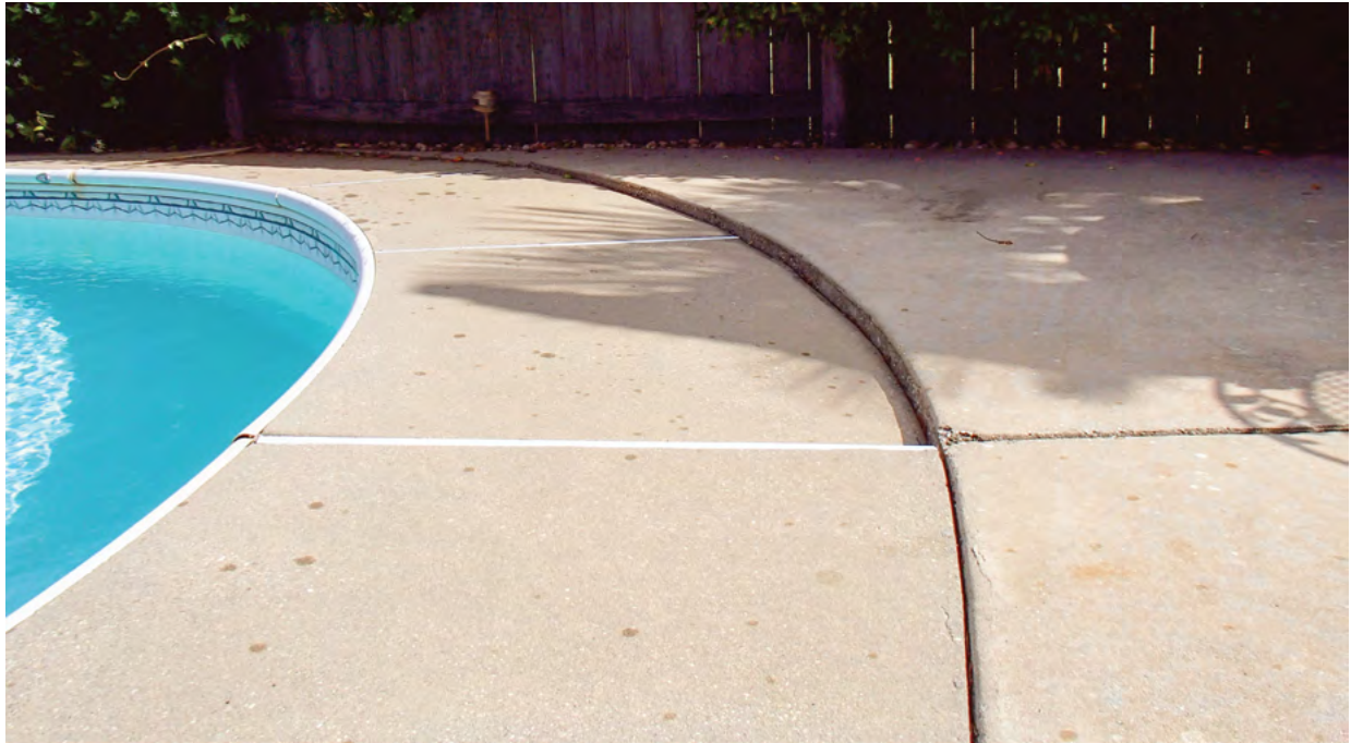
Figure 5.5 Pool deck slab settlement
