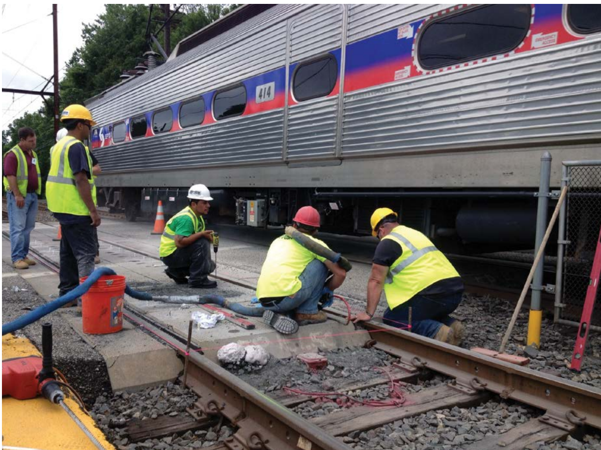
Figure 5.7 Commuter train track settled up to 2 inches at roadway intersection
