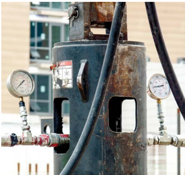
Figure 1.81 Dual pressure gauges
