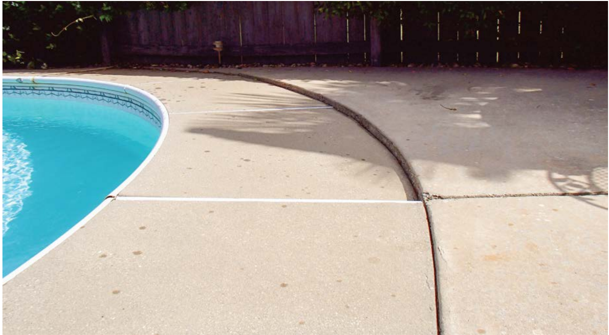
Figure 5.5 Pool deck slab settlement
