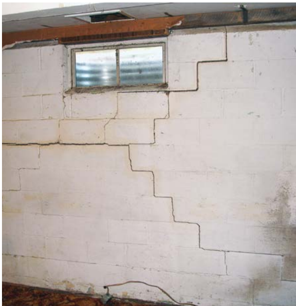
Figure 3.1 Typical stair step crack pattern on a bowing CMU wall
