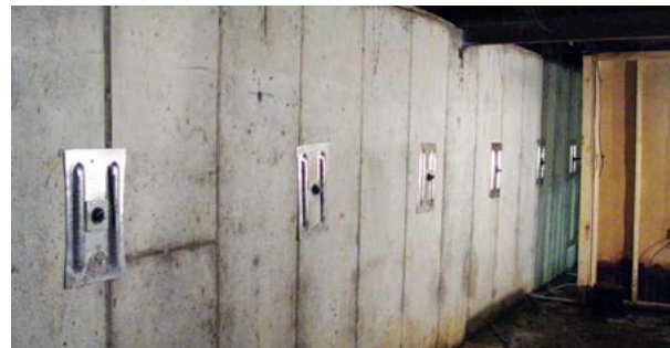
Figure 3.10 After: Wall is immediately returned to original straight position after backfill soil is removed and GeoLock anchors installed
