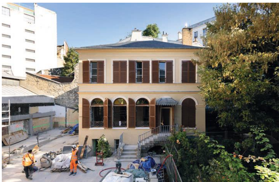
A view of the Musée de la Vie Romantique undergoing renovation works in September 2025
