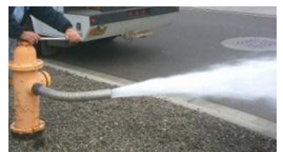
Routine maintenance such as hydrant flushing (pictured above) and valve exercising helps ensure water quality from the source to your tap.
